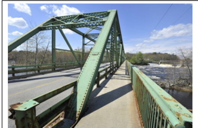
One high-priority project is the Bar Mills Bridge carrying Route 4A over the Saco River at the Buxton-Hollis line.
