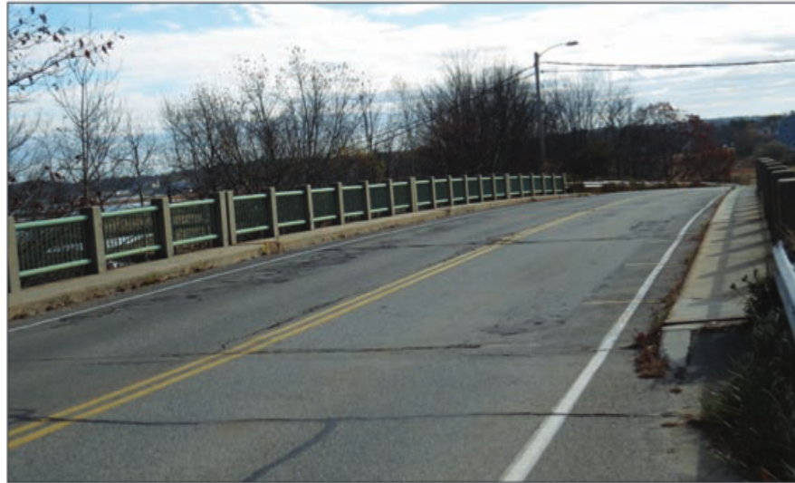
A federal transportation advocacy group has listed the Pine Point Crossing Bridge as one of its top transportation concerns in the state and recommends the bridge gets replaced. The Maine Department of Transportation has the project in its three-year work plan. (Michael Kelley photo)
