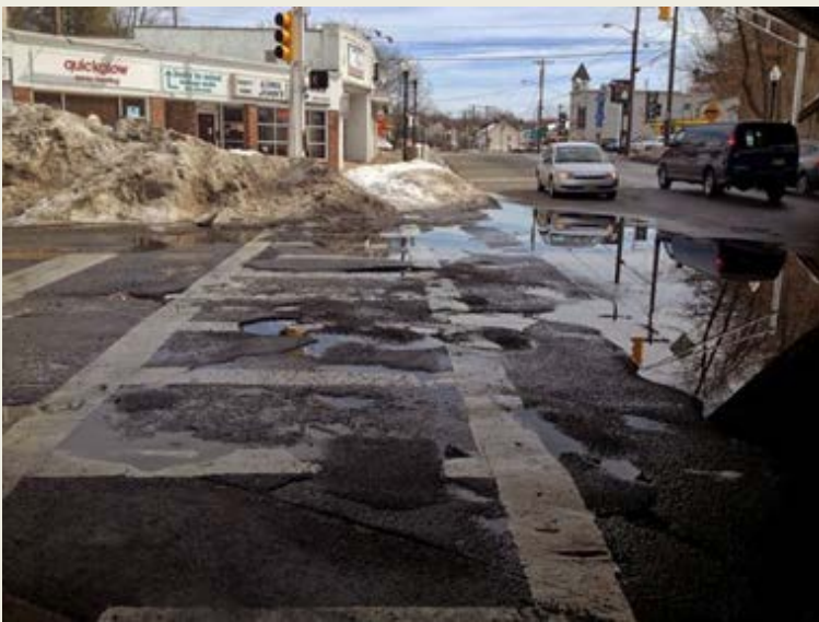
A series of potholes under the train trestle on Morris Street in Morristown was a casualty of New Jersey's rough winter last year of freezing cold, rain and snow followed by the occasional warm day. (Photo: file photo)
