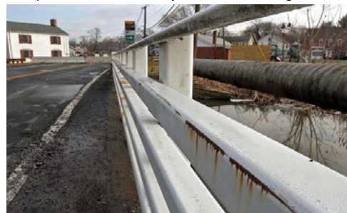
The Amwell Road bridge over the Delaware and Raritan Canal was closed last week for emergency repairs. Repairs
