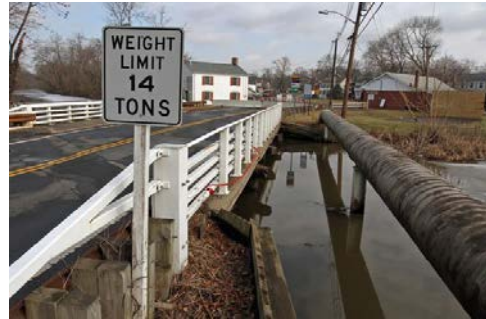
The Amwell Road bridge over the Delaware and Raritan Canal was closed last week for emergency repairs. Repairs are expected to take through the end of February. (Photo: Kathy Johnson/Staff Photographer)
