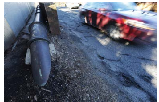
Vehicles travel over the Morris Avenue Bridge which spans over NJ Transit rail lines and is in need of repair. Summit, NJ 1/13/15 (Robert Sciarrino | NJ Advance Media for NJ.com)
