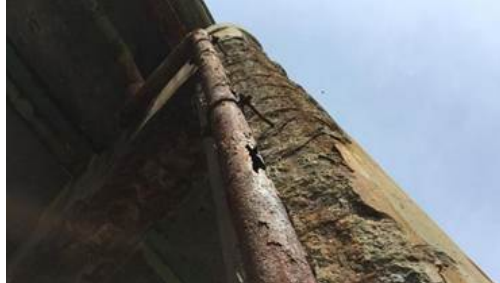
A deteriorating concrete on an overpass on Route 390 over a Gates road last spring. (Photo: File photo 2015)
