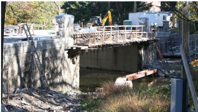
Reconstruction work from earlier this month on the Montebello Road bridge. (Photo: Peter Carr/The Journal News)
