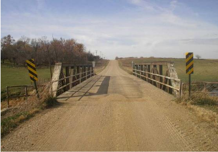
One of the many pony truss bridges that exist across rural Clay County.
