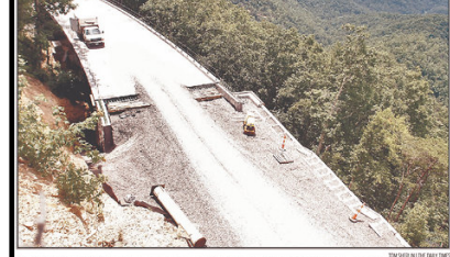
THIS WAS THE SCENE IN 2015 as contractors worked on one of five bridges on the Foothills Parkway between Walden and Weiss Valley.
