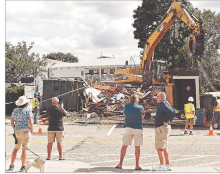
Spectators watch as a crew from Ground Up Construction demolishes the former John's Mystic River Tavern on Cottrell Street in New London on Thursday. The site closed in December of last year, and in January it was announced that the adjacent structure in the main downtown building, The Whisker's Inn also recently demolished the two adjacent residential structures at 1 and 3 Halsey St. Plans have yet to be announced for the site.
