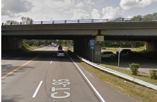
The Interstate 395 bridge over Route 85 in Waterford is the fifth-most heavily traveled "structurally deficient" span in New London County, according to new report released Thursday, Sept. 20, 2018. (Google Street View)
