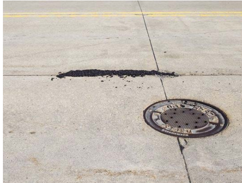
Patched potholes along 10th Street in Port Huron, Feb. 28. (Photo: Brian M. Wells/Times Herald)
