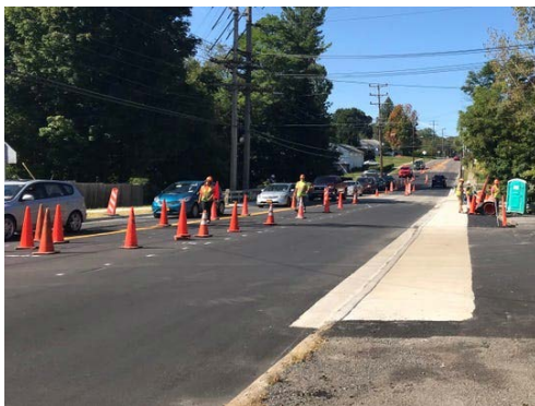
Traffic impacted by construction project on the County Club Road bridge over Patterson Creek Thursday, Sept. 19, 2019. (Photo: Katie Sullivan Borrelli / Press & Sun-Bulletin)
