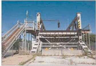
US&J FILE ART The now-closed North Adam Street canal lift bridge is one of seven bridges in eastern Niagara County whose "poor" or structurally deficient condition is cited in a new report by TRIP.
