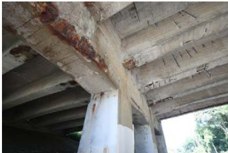
The underside of the Route 100C bridge, above Route 9A in Greenburgh, Sept. 17, 2019. (Photo: Mark Vergari/The Journal News)
