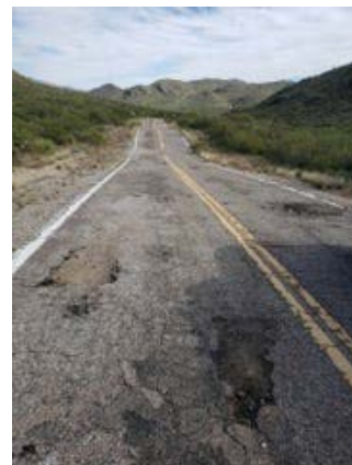
Potholes and rough pavement are nearly unavoidable on Colossal Cave Road in Pima County on Oct. 30, 2019. (Photo: Pima County)
