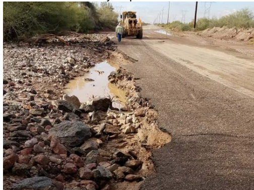
Erosion is eating into the White Wing Wash crossing on Palomas Road near Hyder in Yuma County. (Photo: Yuma County)
