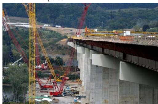
The Central Susquehanna Valley Transportation project (CSVT) bridge across the West Branch of the Susquehanna River in Union Township, Union County. The 4,545-foot-long highway bridge will carry traffic over the Susquehanna River. October 2, 2019. Dan Gleiter | dgleiter@pennlive.com
