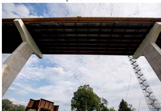
The Central Susquehanna Valley Transportation project (CSVT) bridge across the West Branch of the Susquehanna River in Union Township, Union County. The 4,545-foot-long highway bridge will carry traffic over the Susquehanna River. October 2, 2019. Dan Gleiter | dgleiter@pennlive.com
