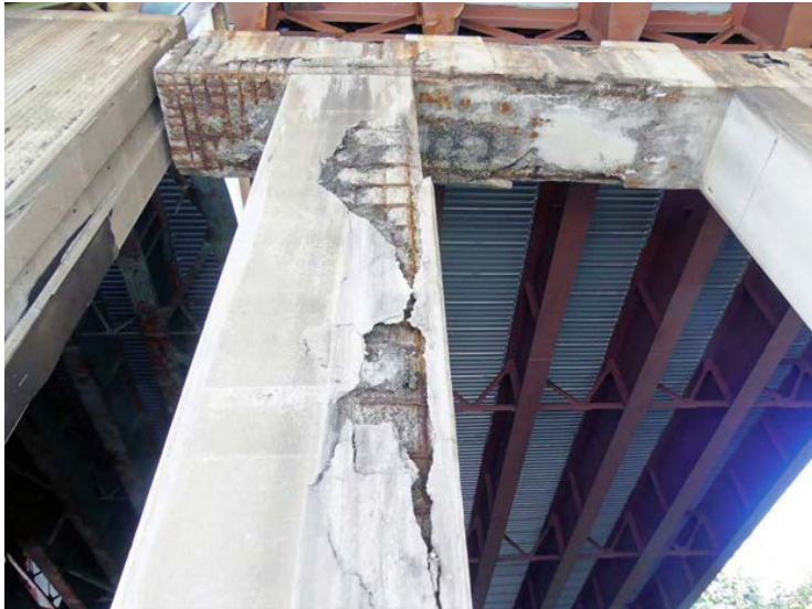
Rebar is exposed on a column of a bridge along the Cross County Parkway in Yonkers.
