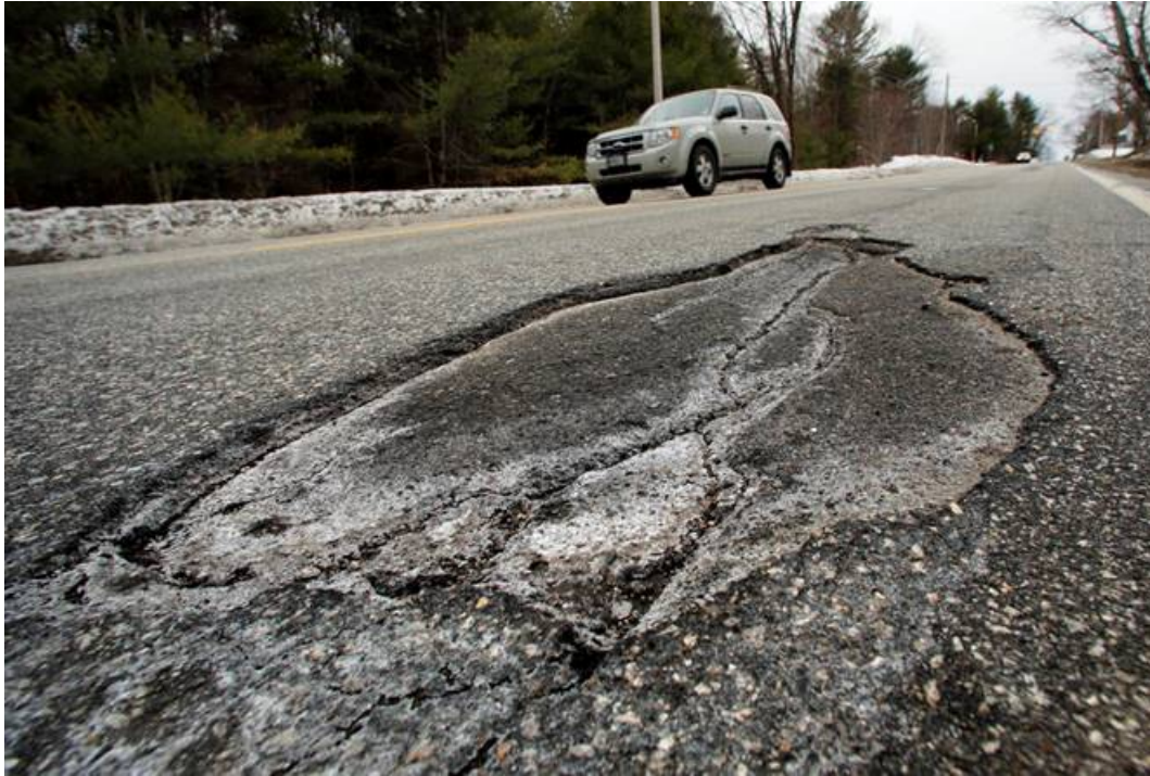
A pothole on Route 302 in Fryeburg in March 2015.
