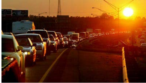
Road work begins Monday at the exit ramps of I-10 at Ambassador. File Photo
