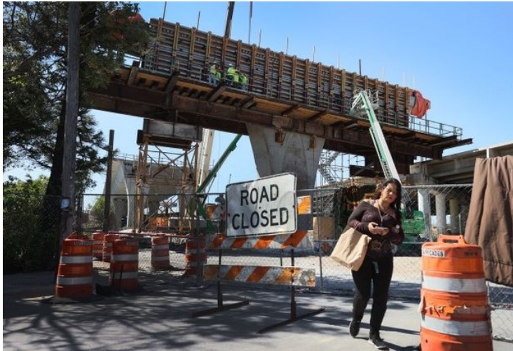
Photographer: Joe Raedle/Getty Images Construction workers build the “Signature Bridge,” replacing and improving a busy Miami highway intersection at I-95 and I-395 on April 13, 2021.
