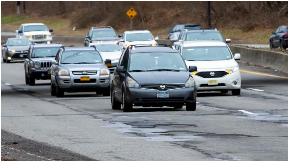
Potholes along the westbound Northern State Parkway in Roslyn in February 2020. Credit: Newsday/William Perlman
