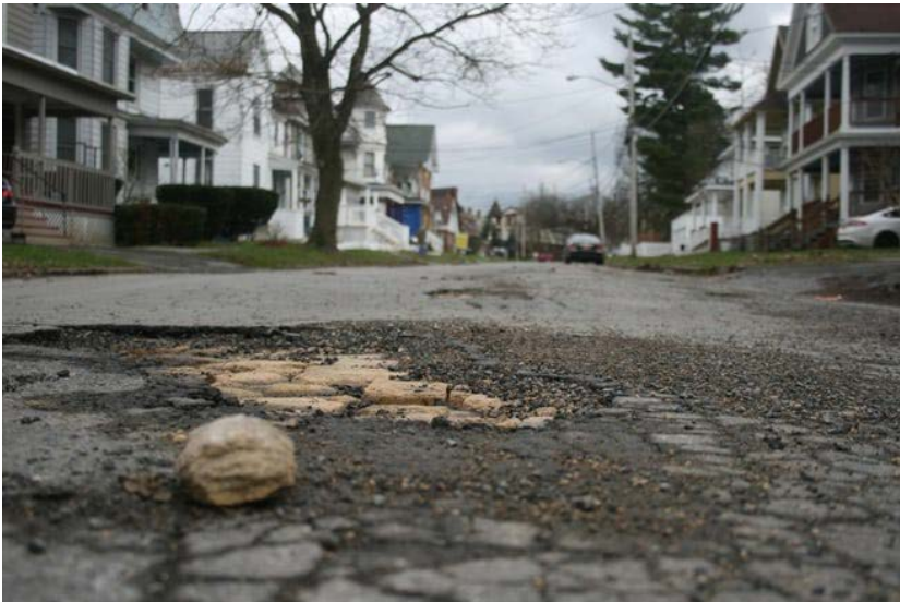
A view of damage to the surface of Shaw Street, east of Sunset Avenue in Utica. STEVEN HOWE / OBSERVER-DISPATCH
