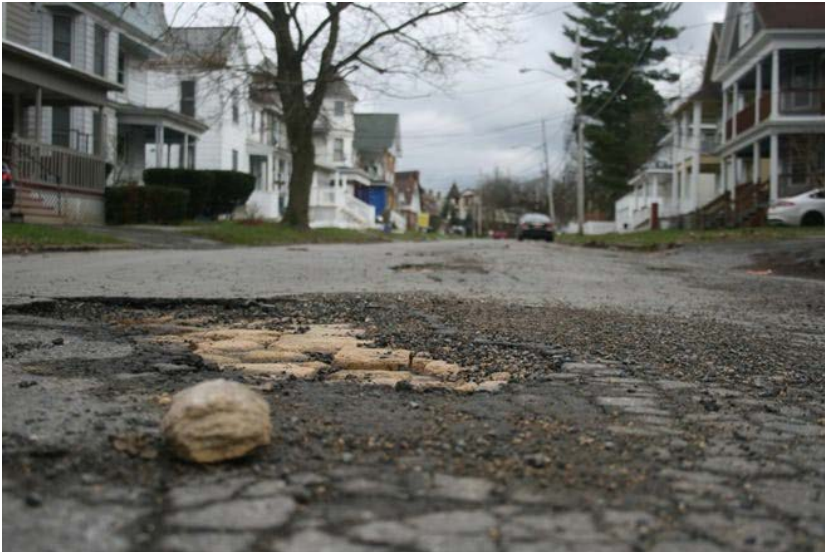
A view of damage to the surface of Shaw Street, east of Sunset Avenue in Utica. STEVEN HOWE / OBSERVER-DISPATCH
