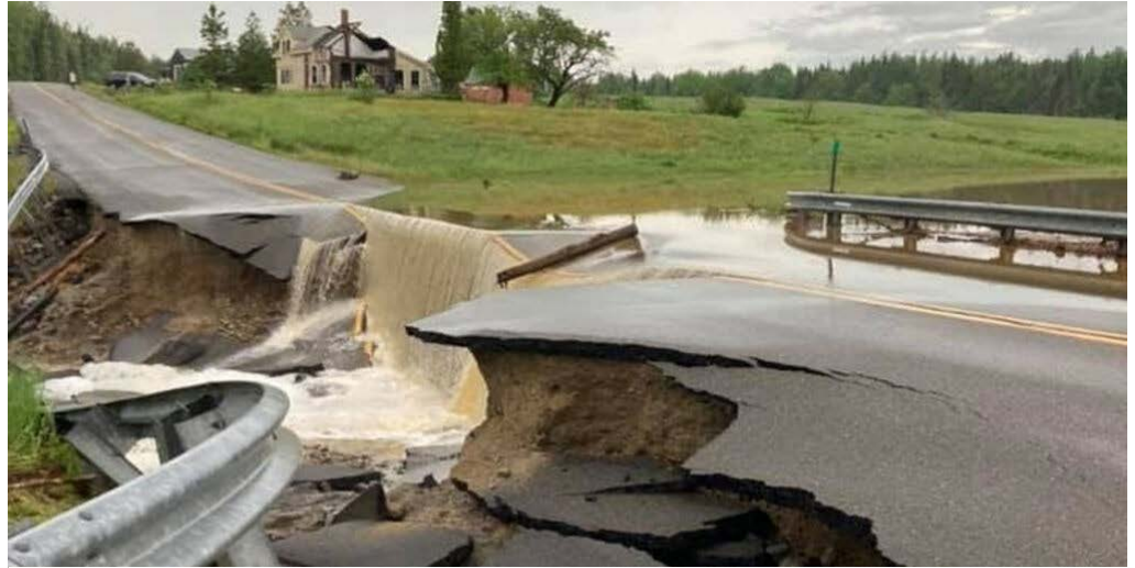
Roads in the Roque Bluffs area in Washington County were washed out in July 2021. (Jonesboro/Roque Bluffs Volunteer Fire Department)
