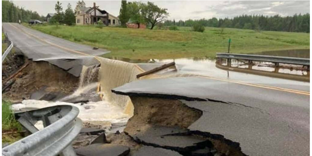
Roads in the Roque Bluffs area in Washington County were washed out in July 2021. (Jonesboro/Roque Bluffs Volunteer Fire Department)
