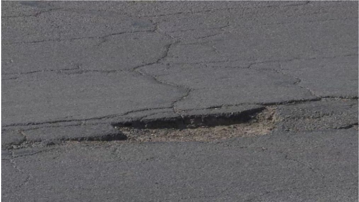
Pothole (Credit: KFOX14/CBS4)
