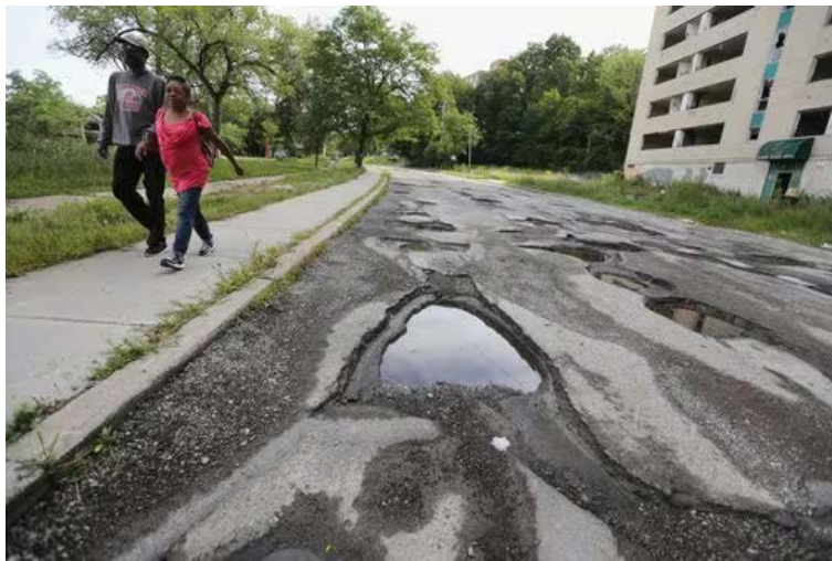
Massive potholes fill with water on Terrace Rd. in East Cleveland. The road was used as an access road during demolition of Huron Rd. Hospital and has not been repaired. The abandoned Huron Place Apartments, right, sit across the street. September 3, 2019 (Gus Chan / The Plain Dealer) The Plain Dealer
