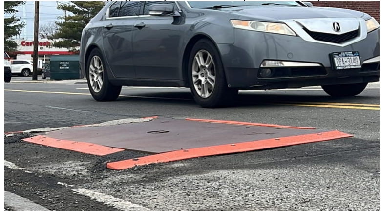
A metal plate covers the North Bellmore pothole in front of a strip mall on Jerusalem Avenue just east of Newbridge Road Wednesday. Credit: Howard Schnapp
