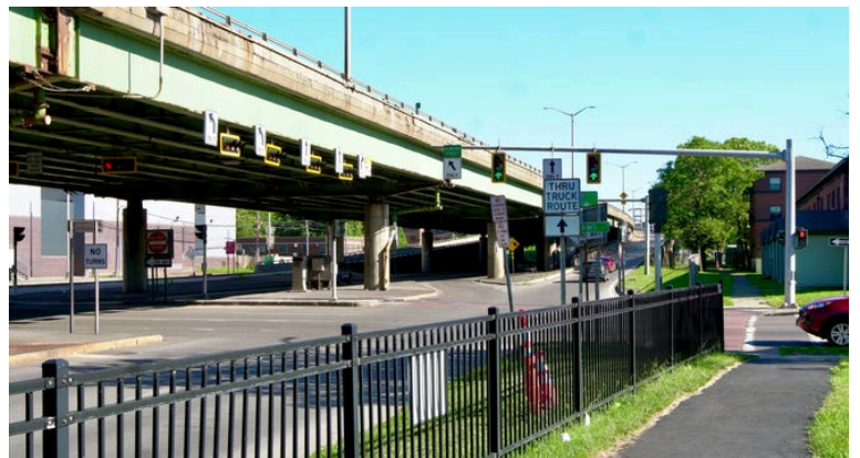
Syracuse's I-81 viaduct is a 1.4-mile elevated stretch that cuts the city in half. On one side is the Pioneer Homes housing project, on the other side is Upstate Medical University. Robert Bell/Rochester Democrat And Chronicle .
