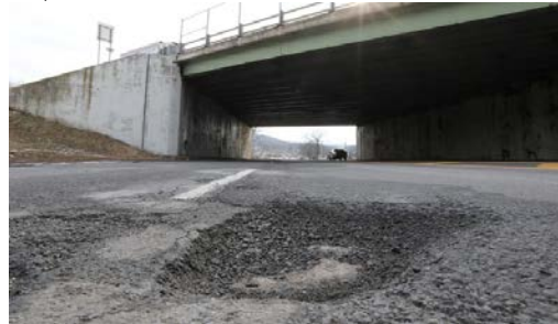
A pothole in the middle of Rt. 303 in West Nyack Jan. 25, 2022. Peter Carr/The Journal News
