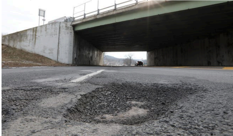
A pothole in the middle of Rt. 303 in West Nyack Jan. 25, 2022. Peter Carr/The Journal News
