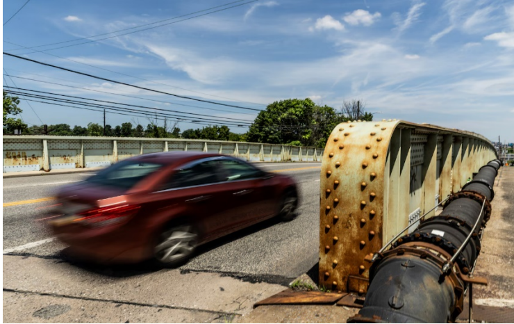
A bridge on Paxton Street in Harrisburg is one of the most heavily traveled bridges in the region that is rated to be in poor condition. June 20, 2024. Sean Simmers | ssimmers@pennlive.com Sean Simmers
