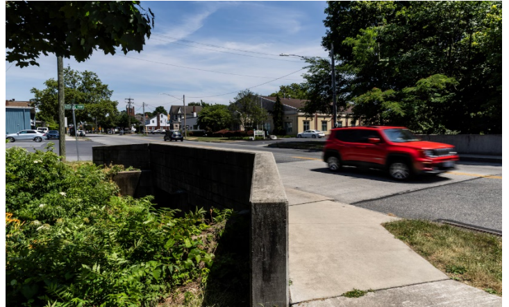
A bridge on Derry and Paxtang Parkway is one of about 10% of bridges in the Harrisburg area that is rated as being in poor condition. June 20, 2024. Sean Simmers | ssimmers@pennlive.com
