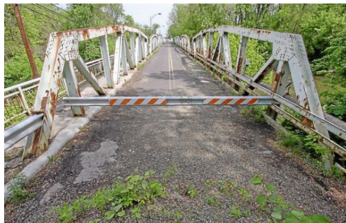
The Keim Street bridge was closed to traffic in 2010 after being found to be structurally unsound. It was recently listed in a report to be among the region's most unsafe bridges. (MediaNews Group File Photo)
