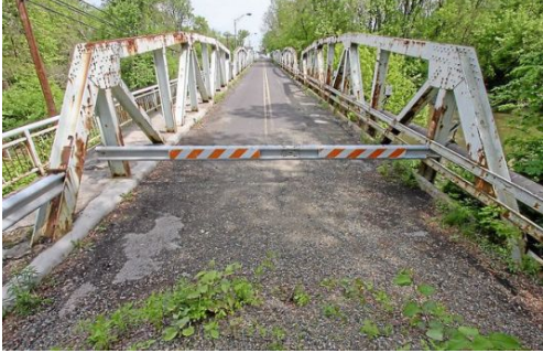
The Keim Street bridge was closed to traffic in 2010 after being found to be structurally unsound. It was recently listed in a report to be among the region's most unsafe bridges. (MediaNews Group File Photo)
