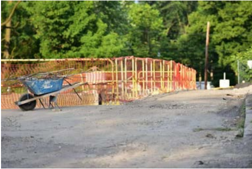
The Parker Street bridge in Scranton is currently having work done. CHAD SEBRING/STAFF PHOTO
