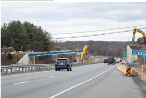
A bridge carrying Suscon Road over Interstate 81 in Pittston Twp. under construction on Jan. 26, 2023. TIMES-TRIBUNE FILE JOSE MARCANO
