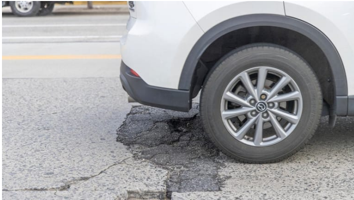
A pothole on Merrick Road outside Bellmore Towing & Complete Automotive Repair in Bellmore on Friday. Credit: Newsday / Howard Schnapp
