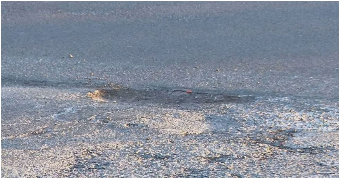
Pothole on a Montgomery County, Maryland, road on Feb 13, 2026. (Mike Rudd/7News)
