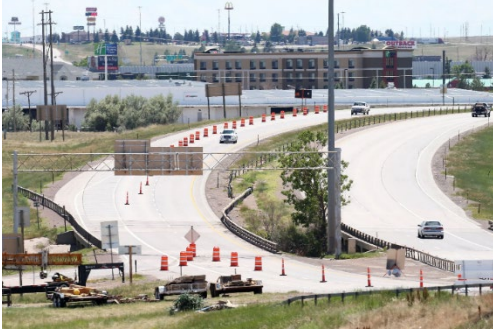
Workers make repairs to concrete slabs along Interstate 25 near Cheyenne in June 2020. Wyoming Tribune Eagle/file
