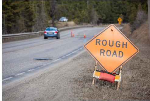
A mild spring in 2025 resulted in potholes developing throughout the Gallatin Canyon, obstructing the roadway. PHOTO BY JACK REANEY
